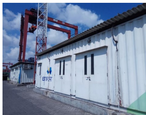
Figure 3. Powerhouse of the shore connection electrical installation
