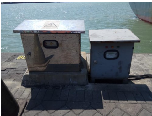
Figure 2. Electric Panel at the dock of BJTI Port
